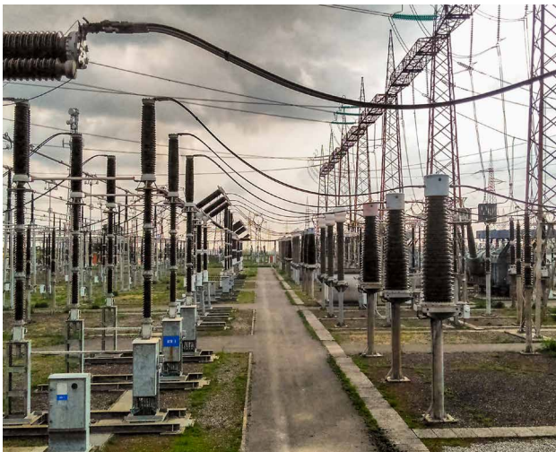
Figure 1: Electrical energy transmission and distribution systems feature a wide range of electrical connections which have a direct influence on the safety of the system.
