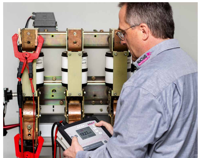
Figure 2: Static resistance measurement on the interrupter units of a medium-voltage breaker with PROMET SE.
