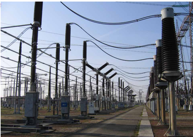
Fig. 1: Switchgear devices are constantly exposed to external factors, such as dirt, moisture and temperature fluctuations, which can have negative effects. Often they are not operated for years at a time and then have to operate reliably under fault conditions.
